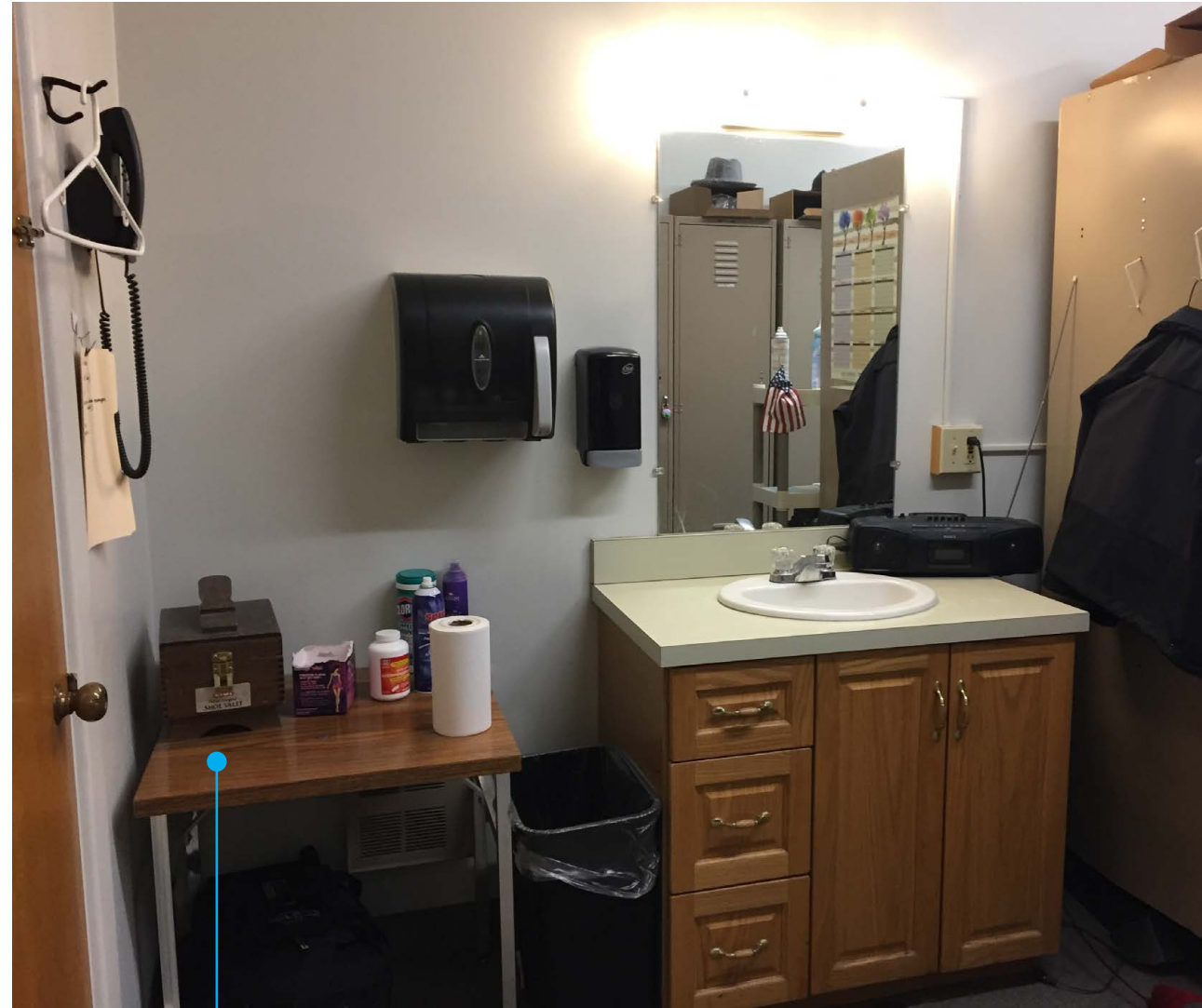
LOCKER ROOMS: LACK OF SPACE AND VENTILATION; STORAGE AND SINK SITUATION ABOVE MORE "TEMPORARY" SOLUTIONS; CARPET FLOORING NOT APPROPRIATE IN WET AREAS.
