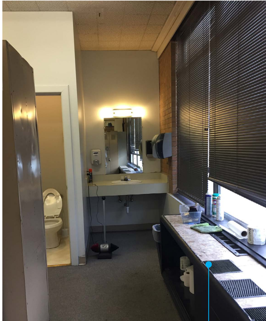
LOCKER ROOMS: NO AIR CONDITIONING (FULL-TIME HEAT BOILER SYSTEM); LACK OF VENTILATION; CARPET NOT IDEAL FOR FLOORING MATERIAL, ESPECIALLY NEAR WET AREAS.
